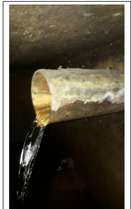
This is the pipe that channels water from the underground to the reservoir. The diameter is 9cm. According to his assessment, we need 2 metallic pipes, 3 pipes with corners, 2 rolls of pipe seal, some spanners.
