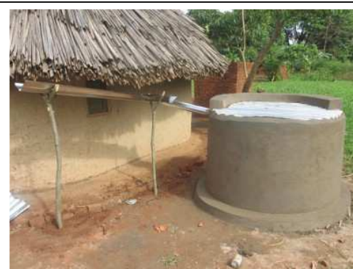
This is the sort of tank that Discover hopes to provide for 50 houses in Kirembe Village, near Kasese, Uganda.
